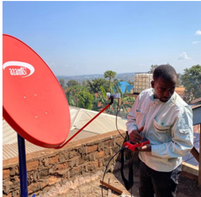
Radio Kwizera technician installing KU Band Satellite transmission on which the radio streams to Karagwe area in Northwestern Tanzania: Photo by Angelo Munduni Dema, SJ
