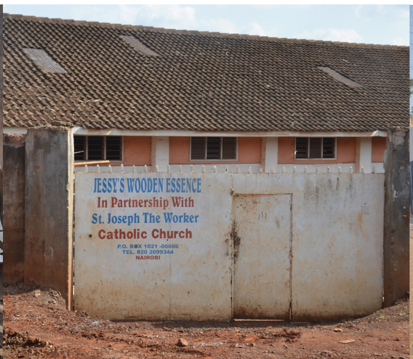
An old gate of what used to be the St Joseph carpentry Workshop
